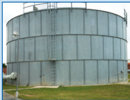
Original Ground Storage Tank at Water Plant #2
